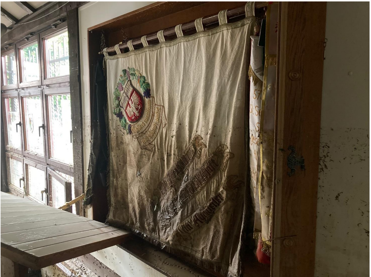
Fig. 2 (bottom): Damaged flag from the museum “Haus der Schützen” in Bad Neuenahr-Ahrweiler which was salvaged with funding provided by Blue Shield Germany
