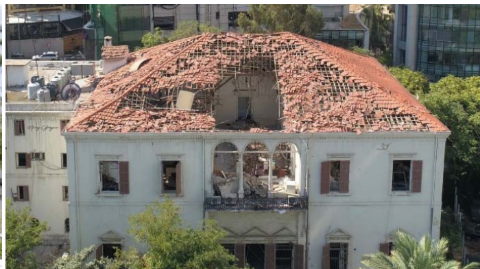
MoFA Building – plot 31 Rmeil AFTER BLAST
