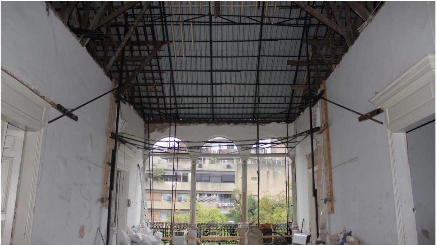
Roof structure and 3 arches held by the propping and bolted into secure walls
