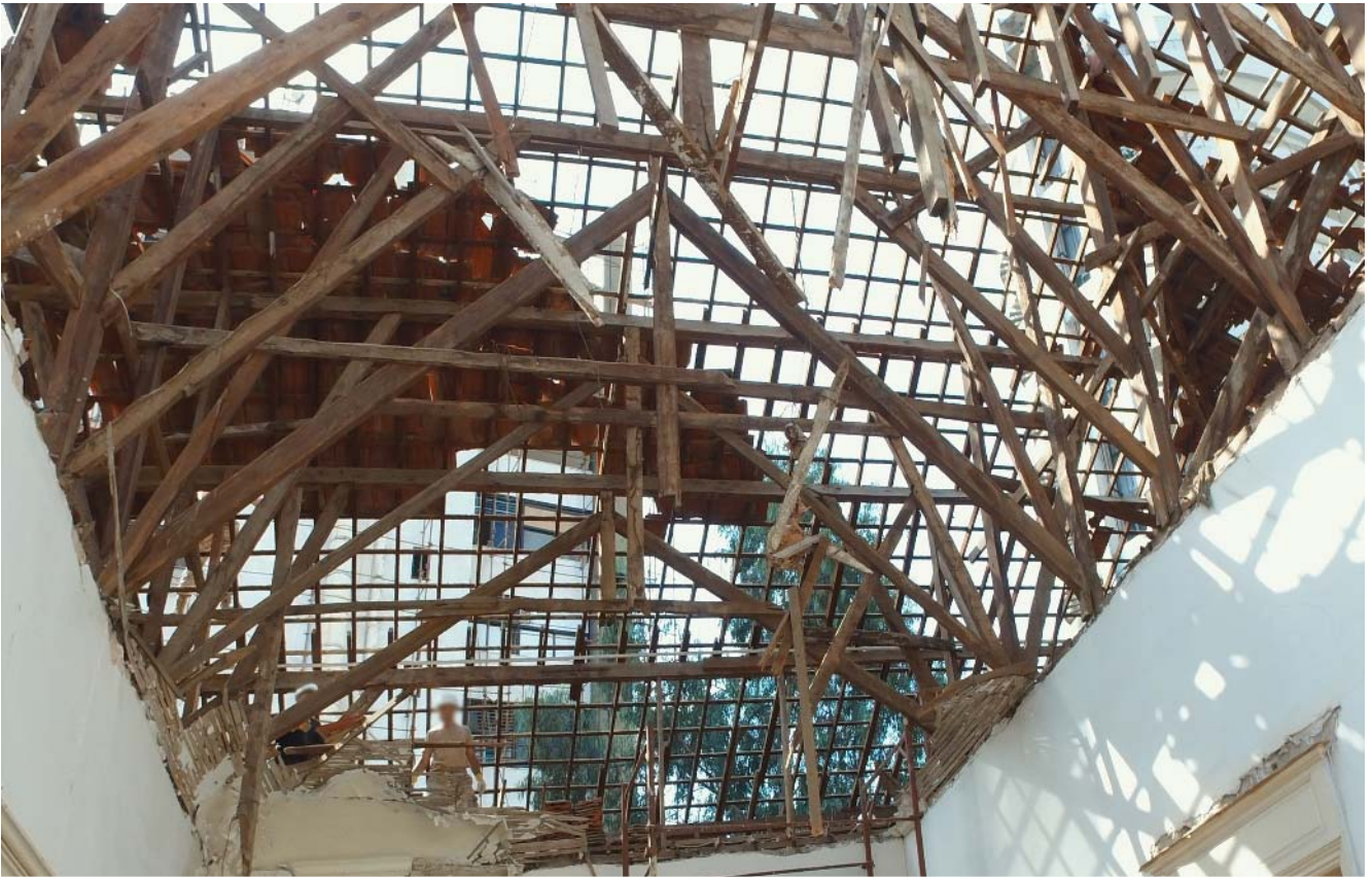
Roof cleared from all rubble and broken tiles
