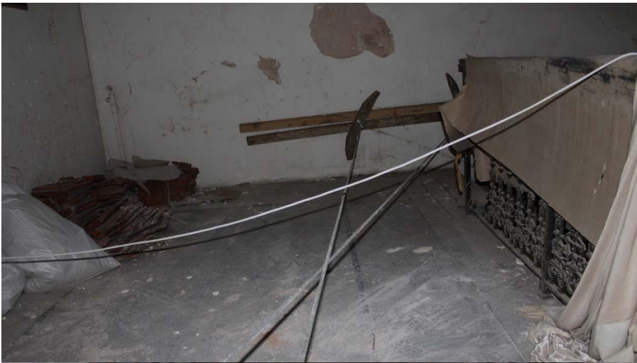
Propping running from wall to wall and fixing the detached wall to more stable areas of the structure and splitting the weight in between all the walls
