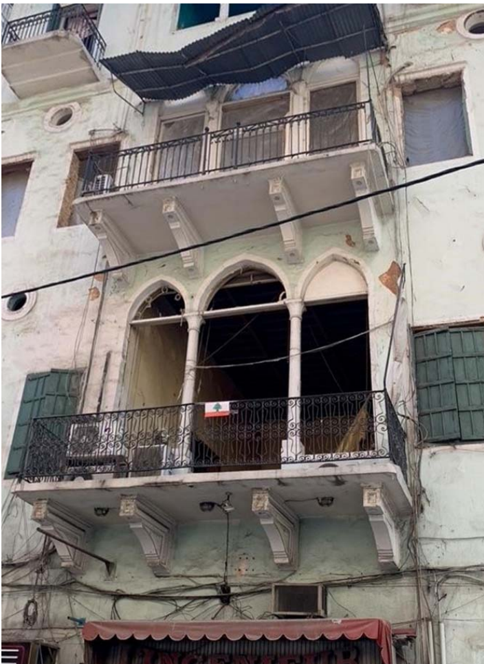
Ghoulam house A – plot 1137 Rmeil AFTER BLAST
